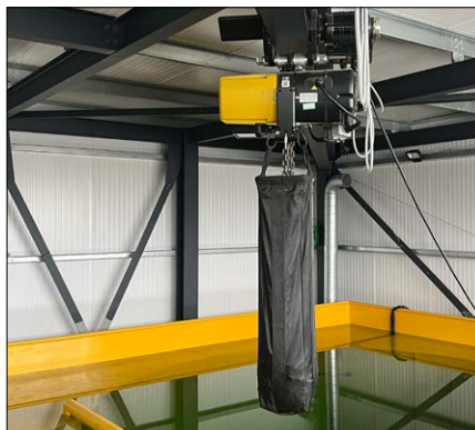
Steel hoist can be used for equipment anchoring and emergency diver recovery.
